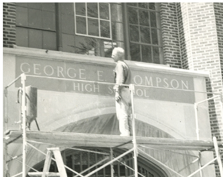
A worker installs the school facade, which is still visible in the main lobby today.
